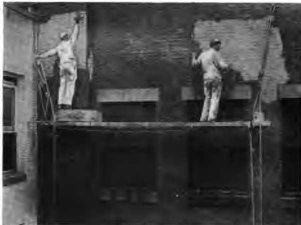
Fig. 2. Unsafe Scaffold Practice.
